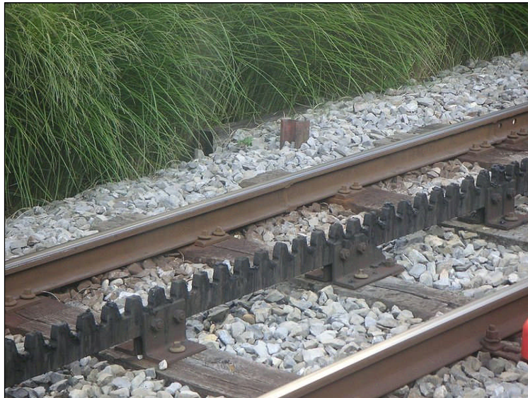
Figure 3.11 – Rail with Rack Bar
