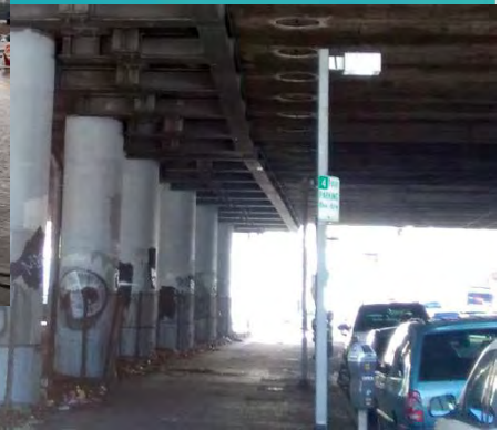
Underpasses have poor lighting and lack basic safety and aesthetic enhancements. People experiencing homelessness are also encamped in the otherwise underutilized space.
