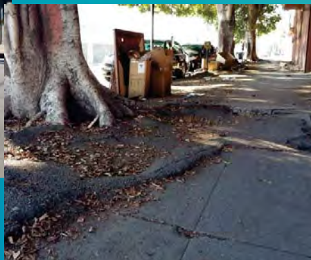
Many sidewalks are broken or uneven, and lack curb cuts with truncated domes. Some areas have no sidewalks.
